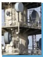
Telecom Data infrastructure
