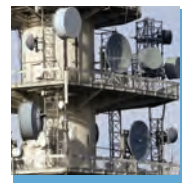
Telecom Data infrastructure
