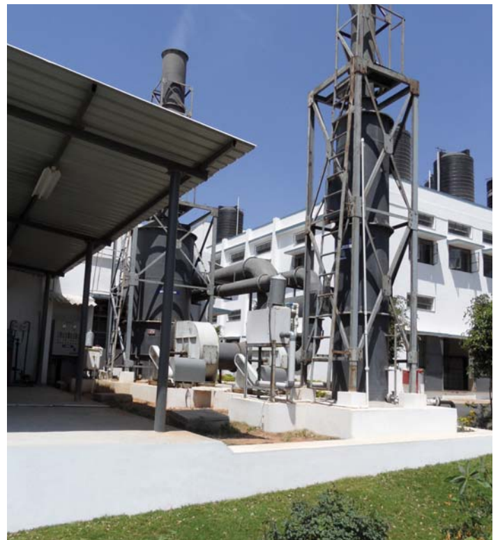
Waste water treatment
